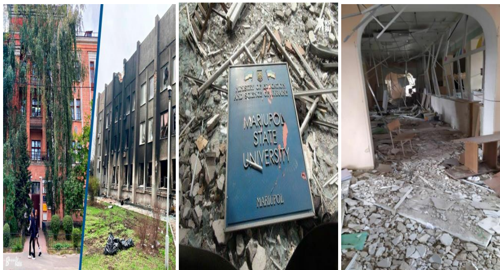
Left – new building of Mariupol State University in Kyiv, Preobrazenska 6, right – ruined building of Mariupol State University in Mariupol (Photo: Natalya Slinkina. https://vechirniy.kyiv.ua/news/71659/ )
